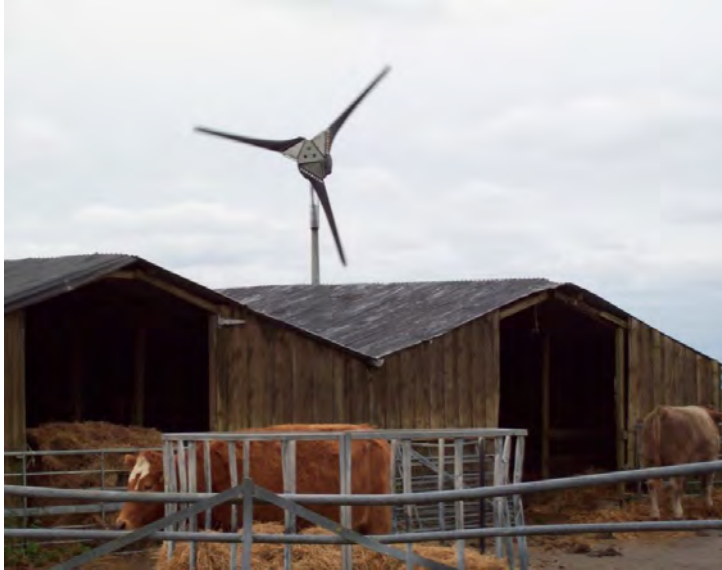
6kW wind turbine
