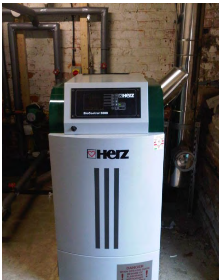
Domestic scale biomass boiler
